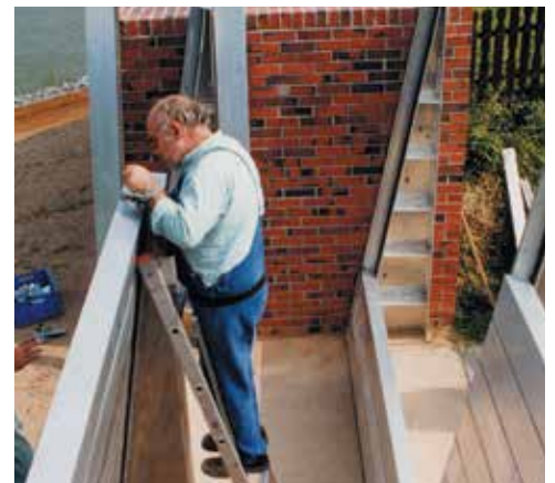
Raising of an embankment in Zons (Germany) – temporary closure of openings in the permanent flood defenses
