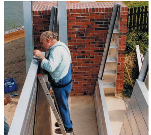
Raising of an embankment in Zons (Germany) – temporary closure of openings in the permanent flood defences
