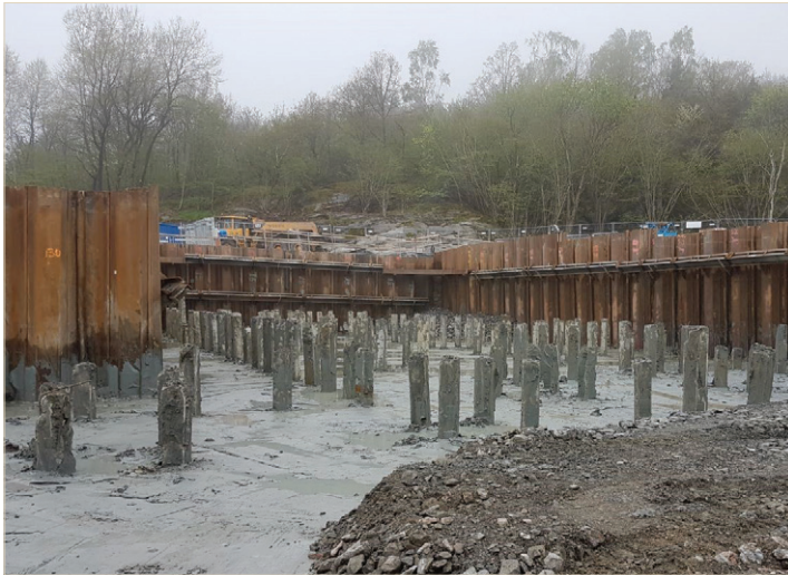
Fig. 5 – Fully excavated pit of building 17. The building is founded on concrete piles.
