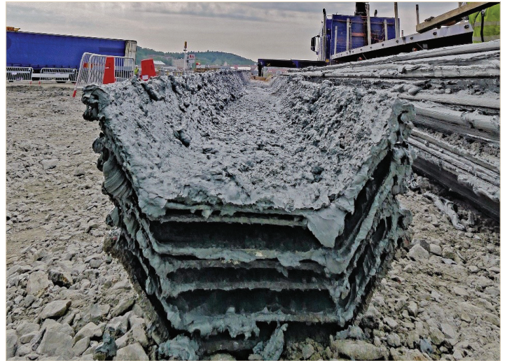
Fig. 8 – Extracted sheet piles that can be reused after cleaning for future projects.
